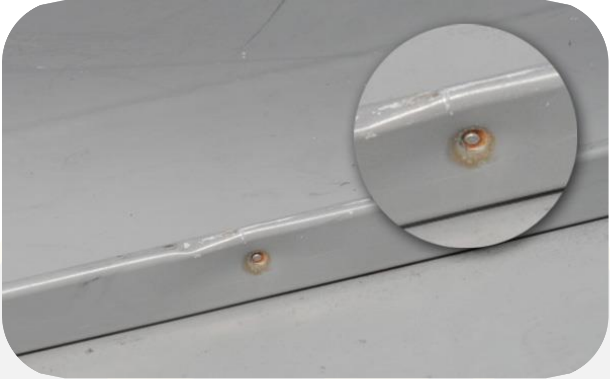
This is the result of cup-point setscrew (competitor part) after 6 years of exposure in the Northeastern U.S. The roof panels had to be replaced.
