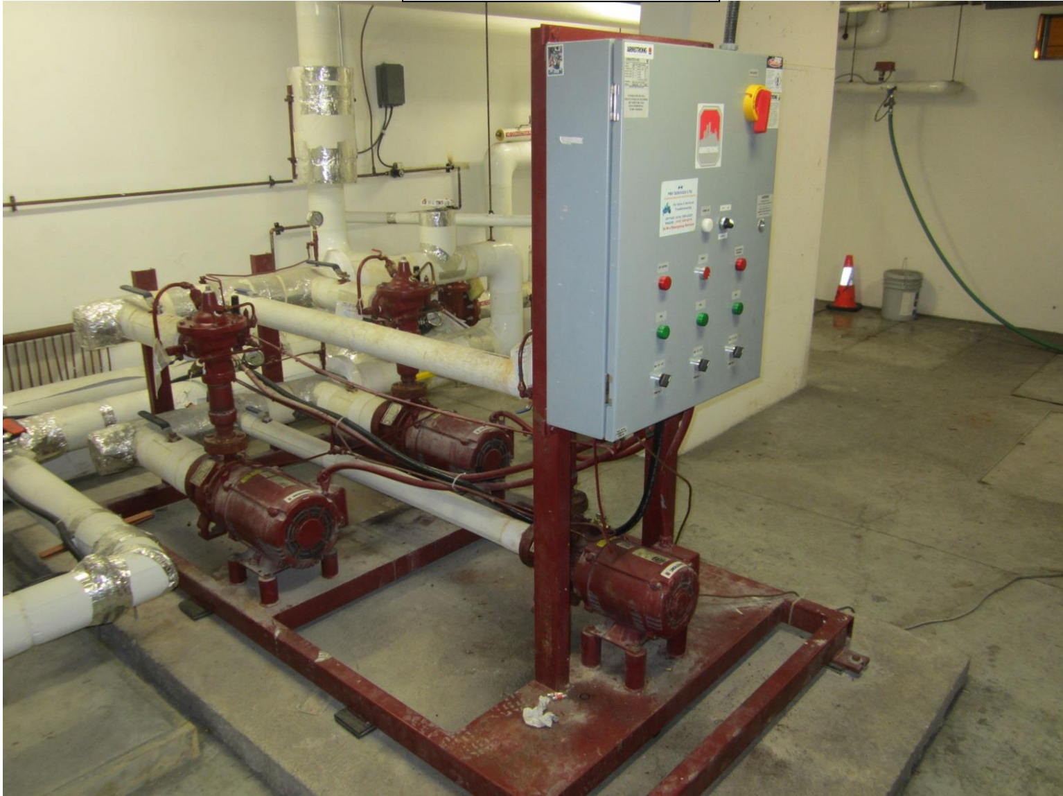
Booster System Picture
