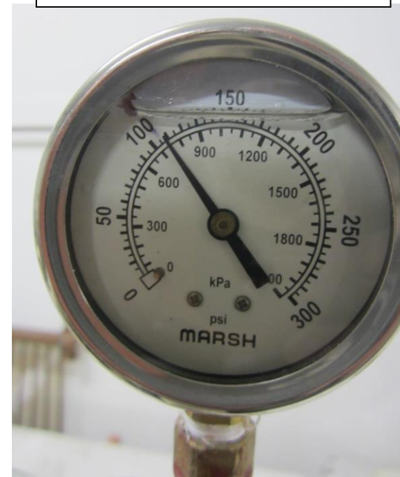
Discharge Pressure Gauge
