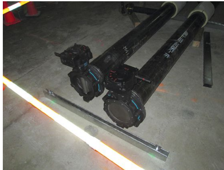
Shown are metal struts for supporting piping systems on slab. Lugged butterfly valves at the chilled water supply and return loops are also visible. Courtesy: ESD
