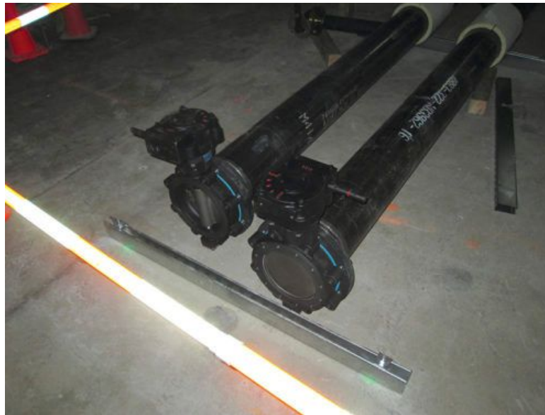
Figure 2: Shown are metal struts for supporting piping systems on slab. Lugged butterfly valves at the chilled water supply and return loops are also visible. Courtesy: ESD
