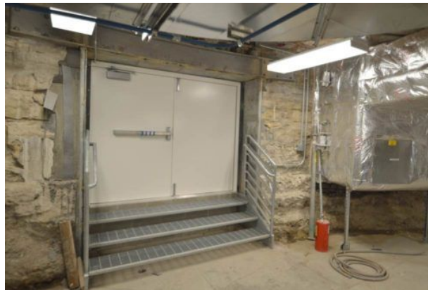
Figure 8: To get the new DOAS unit into Marston Hall's basement, the team designed and installed a new, precisely sized opening in the existing exterior wall. Courtesy: IMEG Corp.
