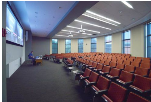
Figure 9: An underfloor air displacement system for cooling and ventilation is employed in Marston Hall's large auditorium, where chilled beams would not be practical. Courtesy: IMEG Corp.
