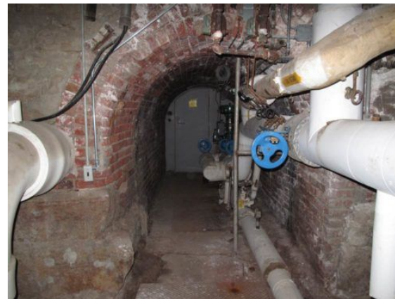
Figure 6: This pre-renovation photo shows Marston Hall's existing tunnel stub looking west. Courtesy: IMEG Corp.
