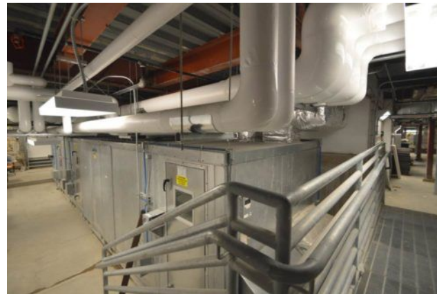
Figure 5: Marston Hall's DOAS unit provides the minimum ventilation air required by code. To the right—above and below the walkway—is the location of the former hot deck/cold deck tunnel. Courtesy: IMEG Corp.
