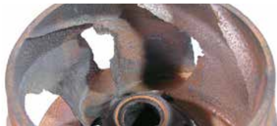
Erosion corrosion of cast iron impeller
