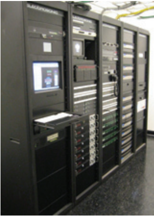
Neat factory-wired racks are always a feature of Electrosonic installations, like these ones at Ford Rouge.
