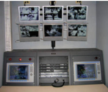
CCTV monitoring system in the ride control room
