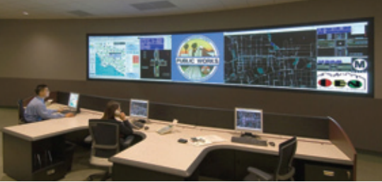
Electrosonic VDS worked with ITS consultant Kimley Horn and contractor MTM Construction when delivering and engineering the display system for the Los Angeles County Traffic Management Center in Alhambra, CA. The system uses Barco 50inch DLP™ XGA cubes, and accepts up to 16 NTSC and four SXGA inputs.
