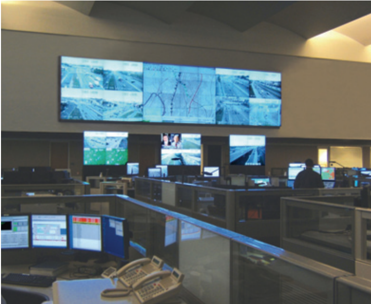
City of Austin (TX) Combined Transportation, Emergency and Communication Center. The display system uses 60 Mitsubishi 50 inch DLP™ cubes.
