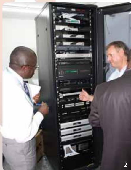
Photograph 1: View from the Control Room. 2: Handing over the equipment rack. 3: The Operations Space. 4: Setting up the complete cabling system for the factory test in Dartford.
