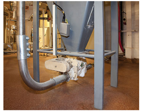
Sugar flows from the floor hopper through a rotary valve into 200 m long PNEUMATI-CON® pneumatic conveying line powered by the blower above the hopper.
