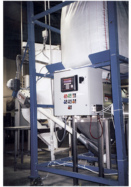
Moistened cornmeal discharged from vertical blender into floor hopper is transported by the Flexicon flexible screw conveyors that feed two extruder surge hoppers.
