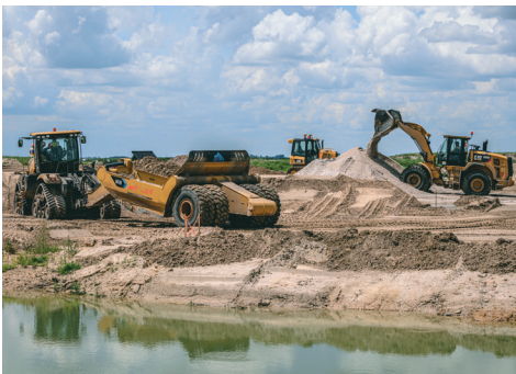
Lane was responsible for construction of the C-43 West Basin Storage Reservoir project, an Everglades restoration effort.
